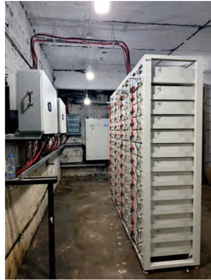
Iraq Warehouse » 100kW+245.76kWh
