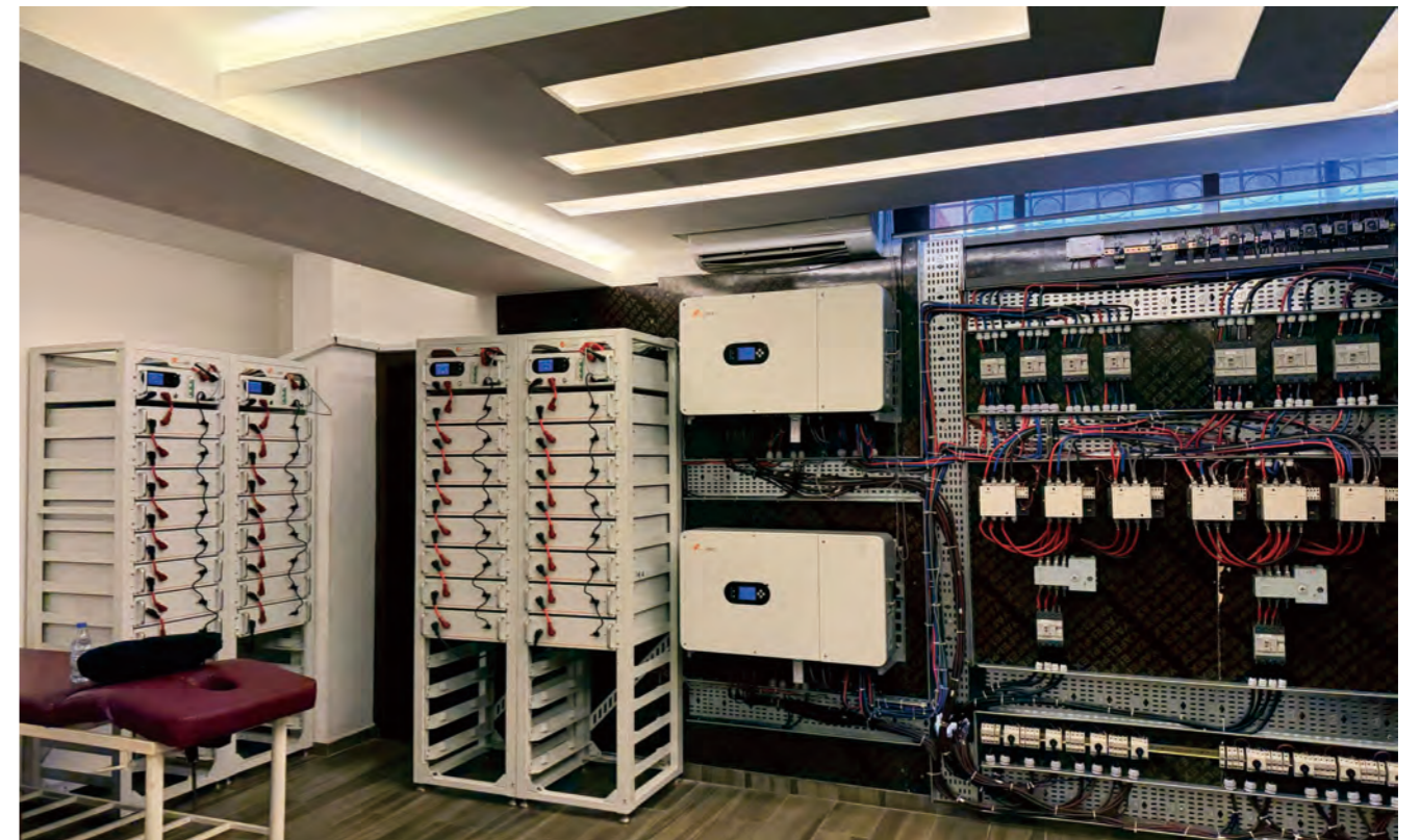
Mexico Hotel » 100kW+163.84kWh
