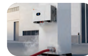
Firefighting External Water Inlet
