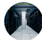
Communication Base Stations
