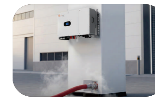
Firefighting External Water Inlet
