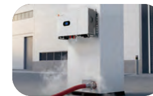
Firefighting External Water Inlet
