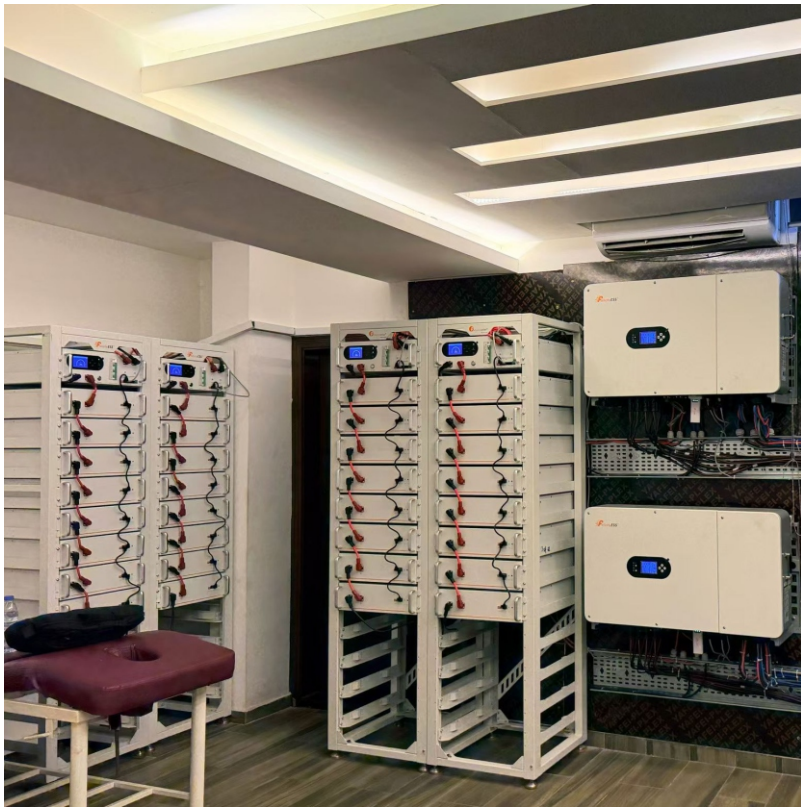
Mexico Hotel 100 kW+163,84 kWh
