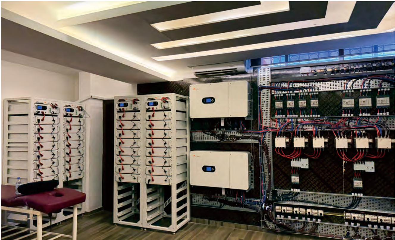
México ➤➤ Hotel ➤➤ 100kW+163.84kWh
