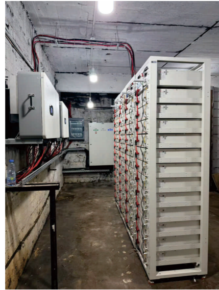
Iraq Warehouse ➤➤ 100kW+245.76kWh
